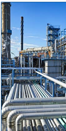
LONG PIPING RUNS WITH HIGH FRICTION LOSS
